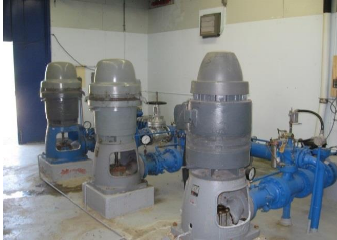
Image 11: Vertical turbine pumps in High Lift Pump Station
