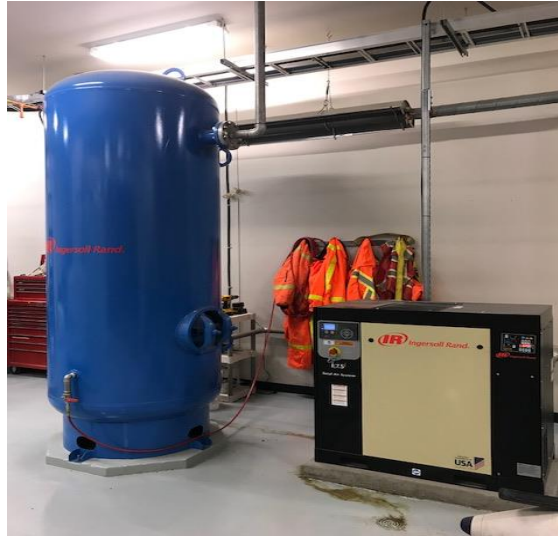
Image 5: Air compressor and tank
