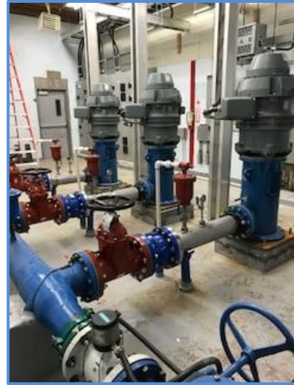
Figure 8. High Lift Pumps
