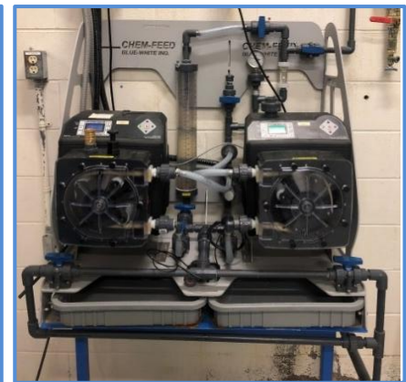
Figure 6. Peristaltic Pumps for Chemical Dosing
