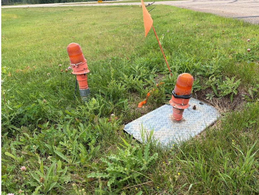
Typical Junction light set up.
