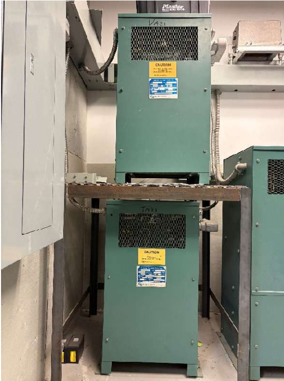
Constant current regulators for taxiway and vasi.
