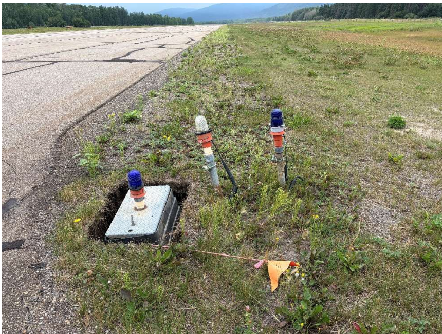
Typical runway light set up at junction of taxiway. Note runway light should be lid mounted, both taxi lights should be post mounted.
